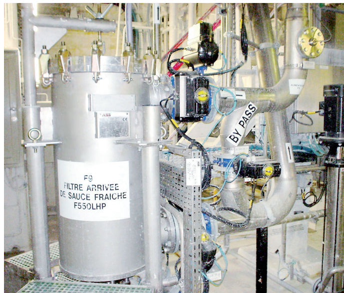
Filtercel LHP F550 installed on fresh colour feeding inlet
